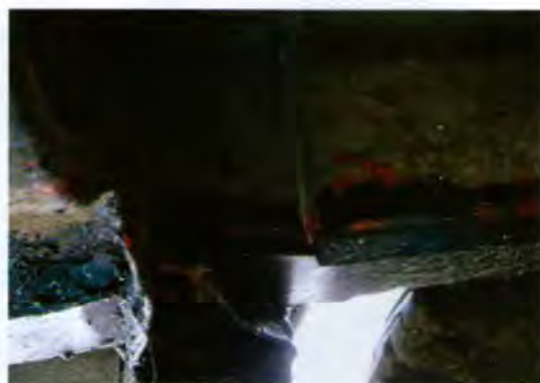
A couple of examples of classic chassis corrosion (above).
