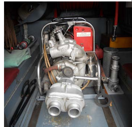
Below: Pump at the ready!
